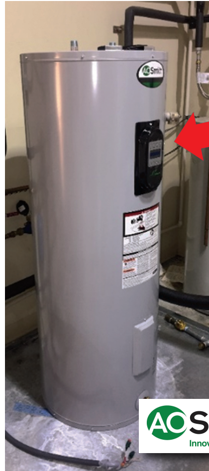
SkyCentrics communication module installed on tank by program contractor
