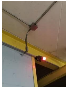
Digester Valve Open Status Indicator light
